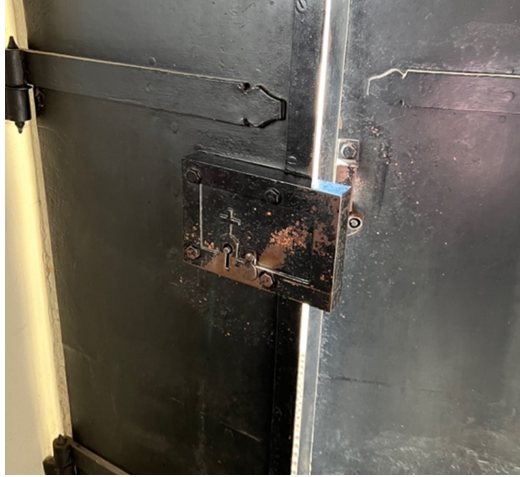
Figure 56. An example of a historic door still functioning in the PoW with the possibility of opening it only from the inside of the building. The Shrine at Jasna Góra in Częstochowa
