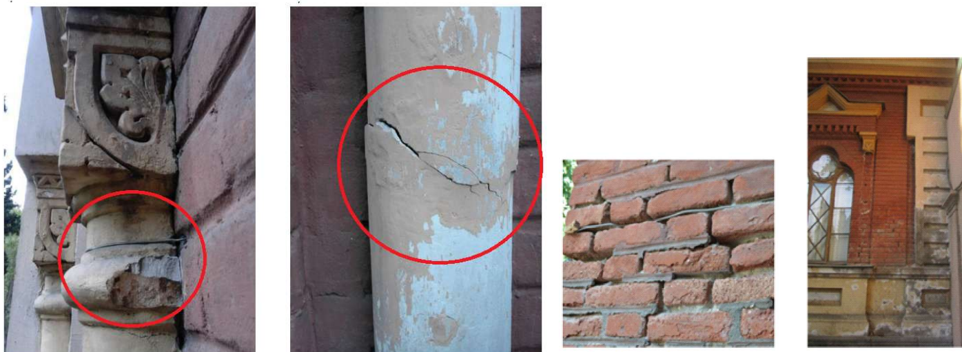
Deteriorated plastered columns on the facade of the State Silk Museum
